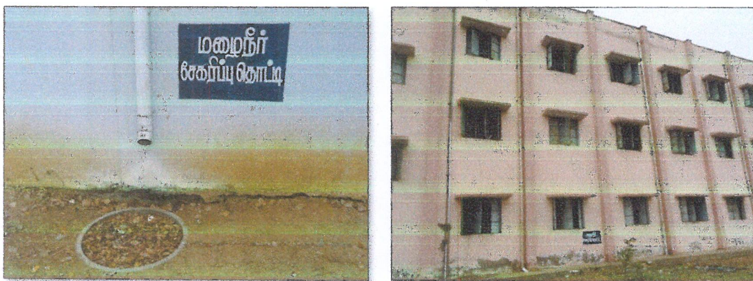
Fig. 5. Rainwater harvesting pit
